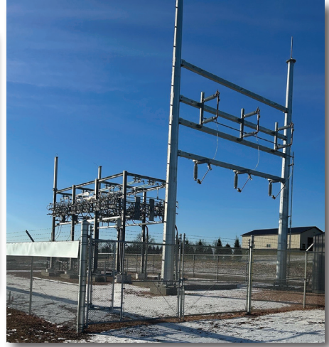
Construction started on the North Wal Substation, located near Wal-Mart in Rice Lake.
