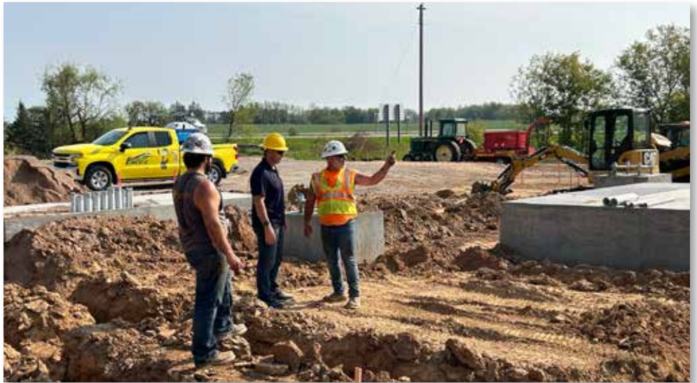
Construction has started on the North Wal Substation, located just north of the Walmart Supercenter.
