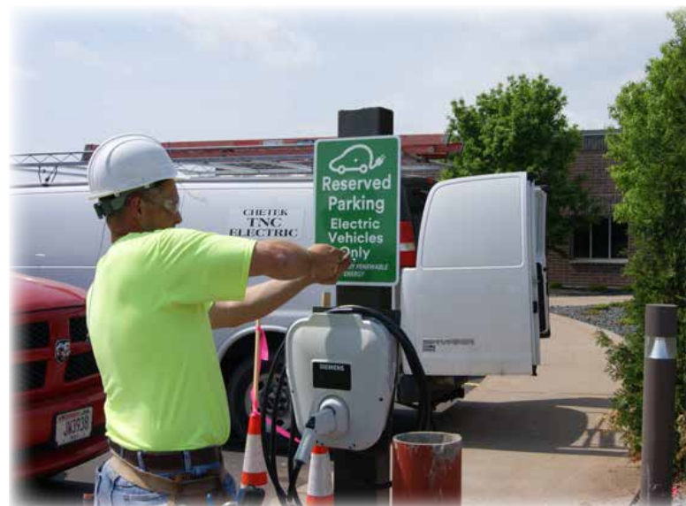
Electric vehicle charging stations were installed at Barron Electric's offices in Barron and Spooner.
